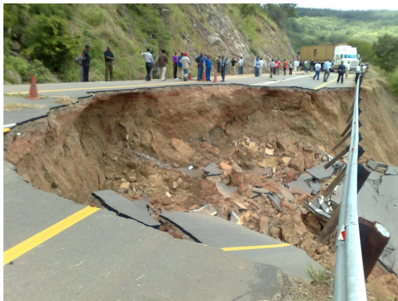
Figure 7: Climate and weather-induced damage to road infrastructure
