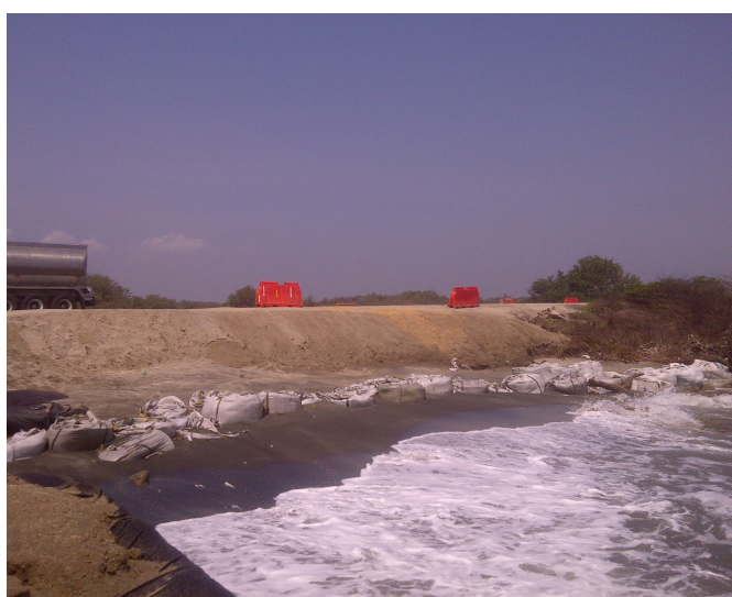
Coastal erosion impacting roads along the Colombian Caribbean. Km 19 Cienaga-Barranquilla. Carmen Lacambra
