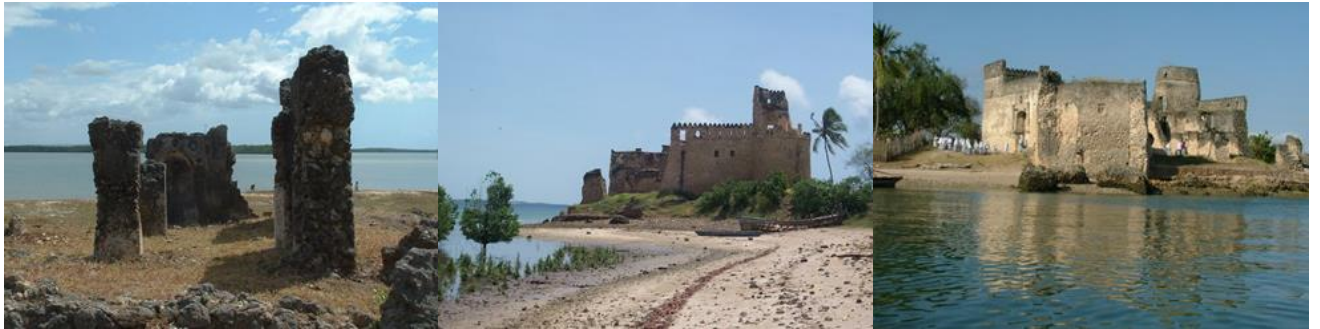
Figure 31: Historical buildings damaged by erosion at Kilwa Kisiwani. Left: location 1. Center and Right: location 2.
